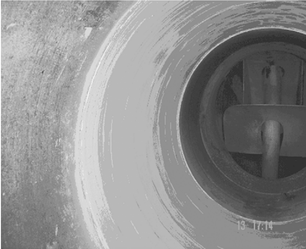
Figure 403-1.1-1 Structural Liner in Raw Water System
